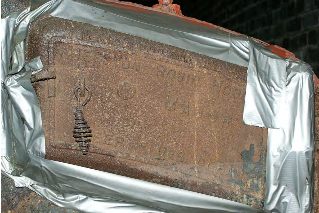
Plate 15: Beeston 'Robin Hood Major' boiler
