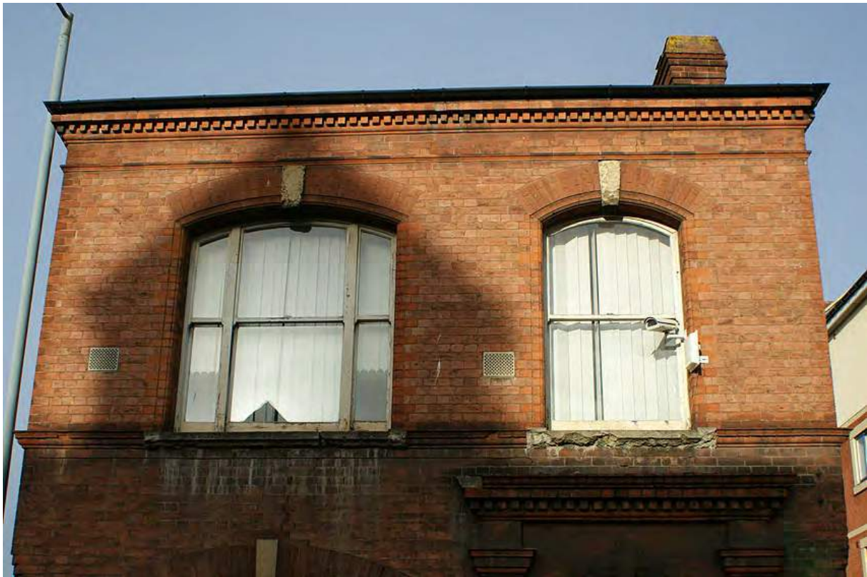
Plate 106: First floor, south elevation of the 'office building' fronting The Butts, showing the eaves cornice, window surrounds and string courses
