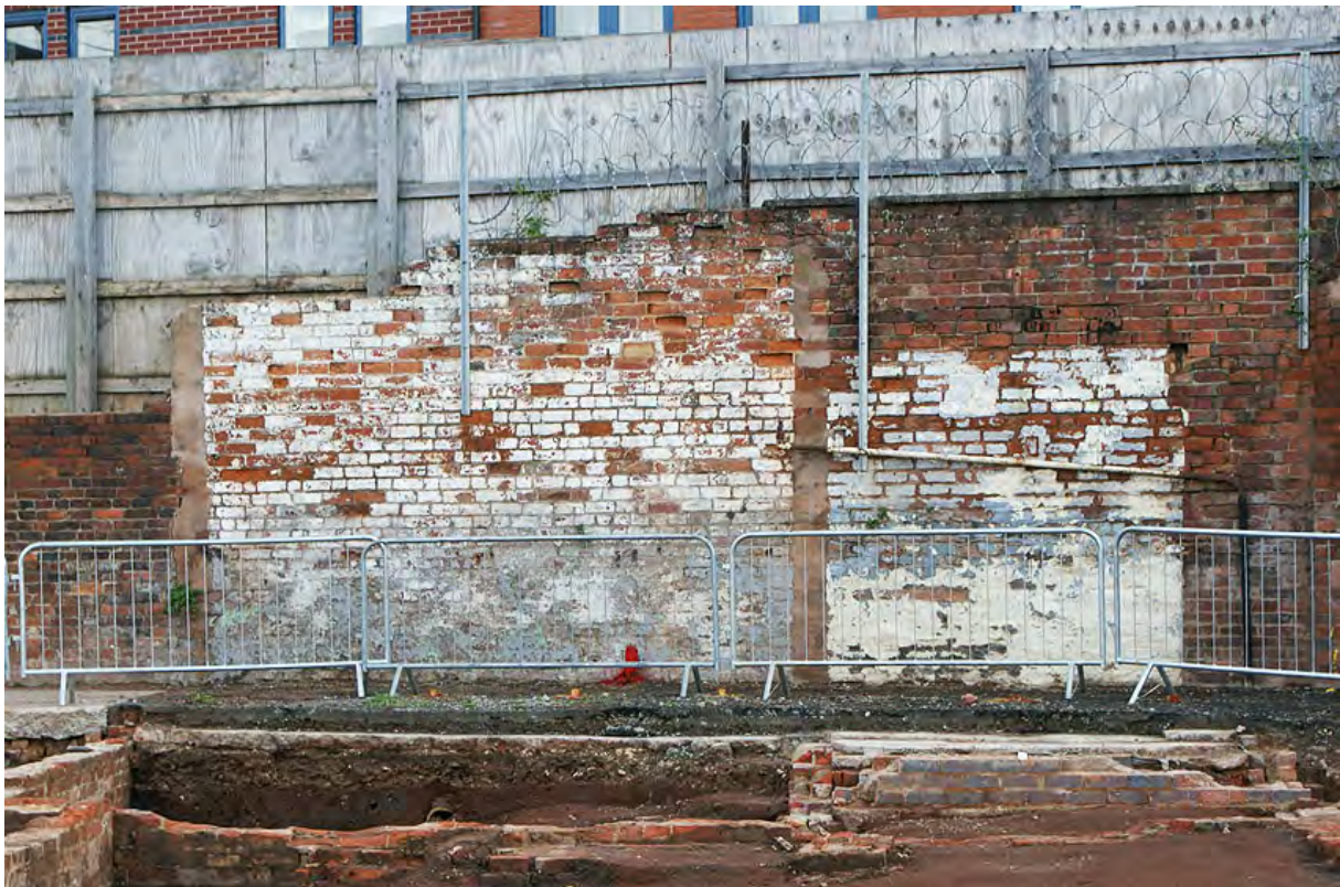
Plate 64: Foundations of range of buildings and the corresponding building scars on the wall
