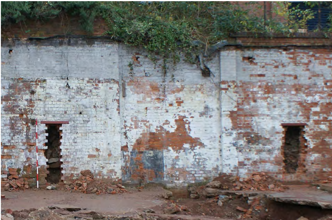
Plate 35: Holes cut into city wall to test the make-up of the wall
