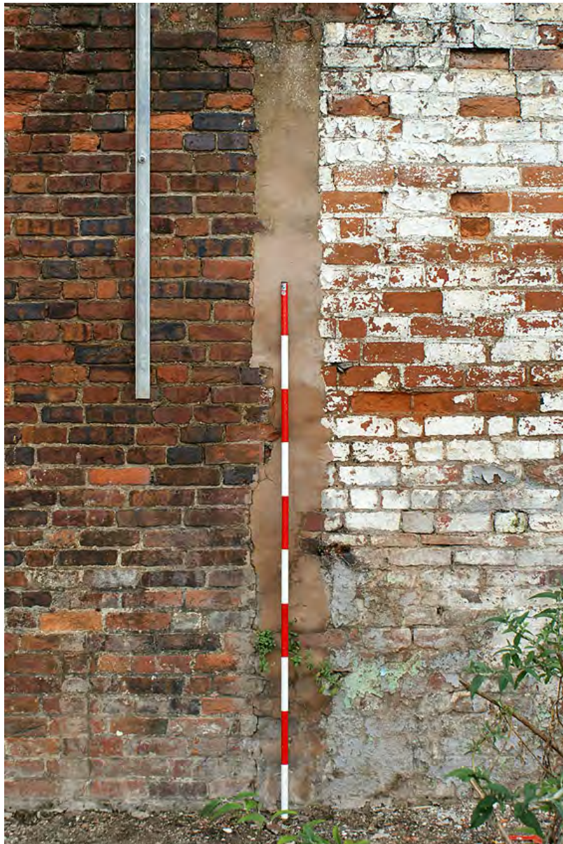
Plate 65: Building scar formed by filling holes with cement
