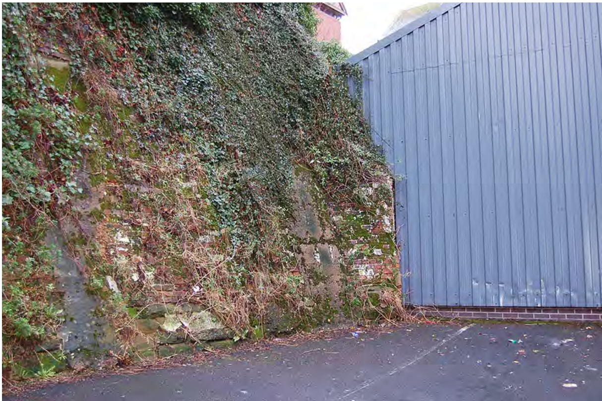
Plate 31: City wall on site adjacent to Transwipers (with Transwipers building on right)
