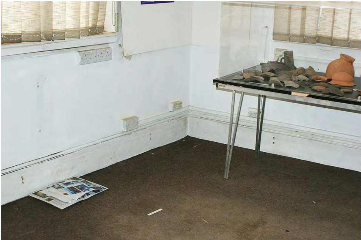
Plate 112: Roll moulded skirting in the building fronting The Butts
