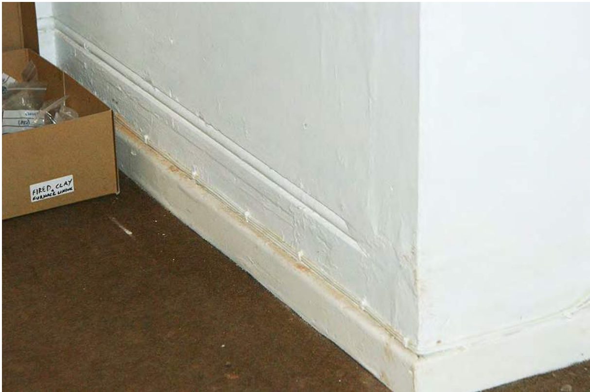
Plate 110: Roll moulded skirting in the building fronting The Butts
