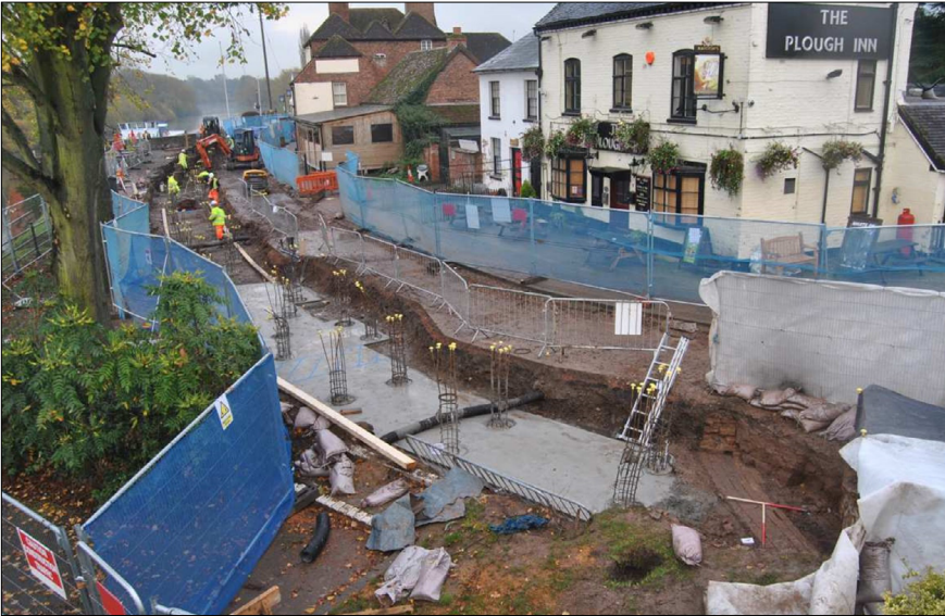
Figure 21: General view of the waterfront from the road bridge, with the curved graveyard wall in the foreground, and the bridges located to the top left, below the working machines; 2m scales; view south-east
