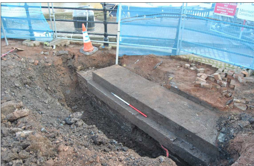
Figure 26: Granite running block (8171) capping the eastern, downstream drawbridge wall; 1m scale; view north-east
